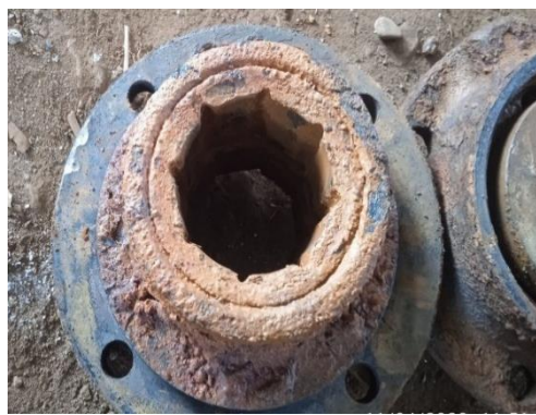
4-rasm. Rezina podshipnikning shikastlangan holati
